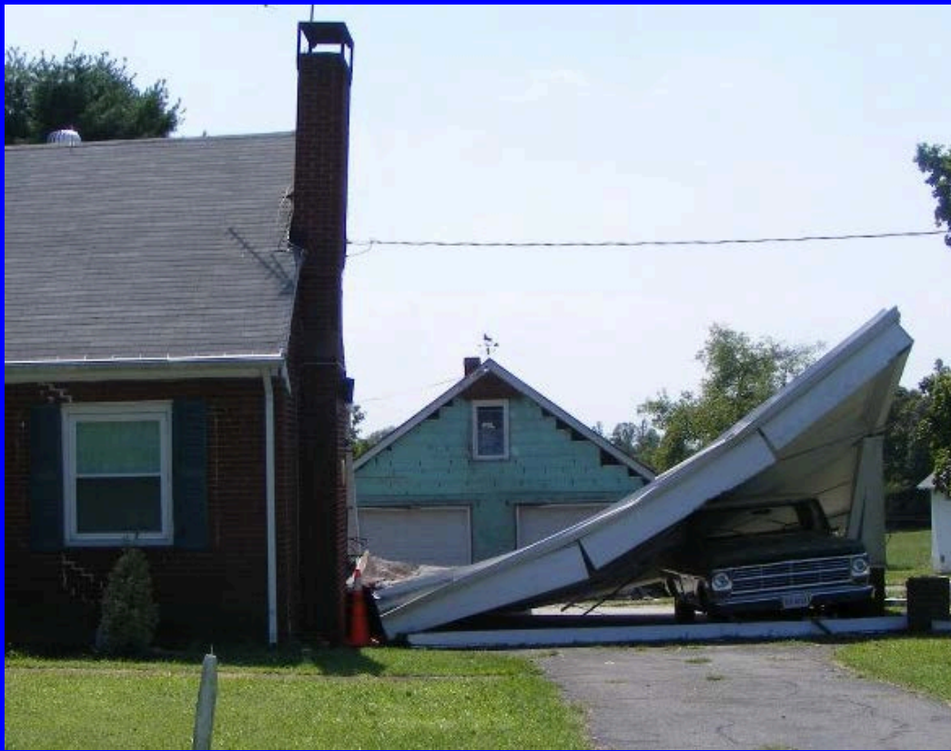
Damage from Aug. 23, 2011 Virginia earthquake From: Bill Barnhart, Cornell grad student
